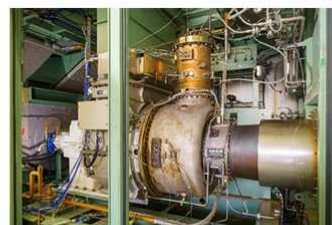
IHI 70% liquid NH 3 cofiring 2MW-class gas turbine, 2020
