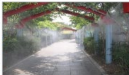
Cooling Fog Facilities
